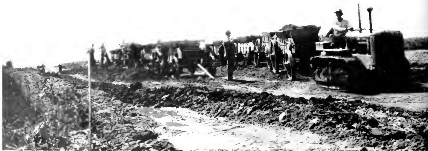
Complying with W.P.A. regulations dirt was moved by wagon trains filled by hand labor and hauled by tractor
